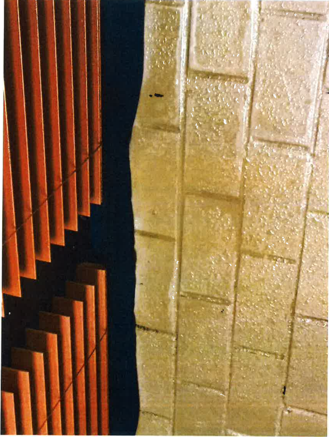
Photo 3: Picture of floor inside of building at front door, showing water blowing in through the storefront, PRIOR to the canopy being installed.
