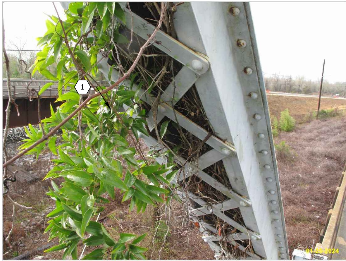
TYPICAL VEGETATION GROWTH ON END DIAGONALS, EAST TRUSS FROM L0-U1 SHOWN
