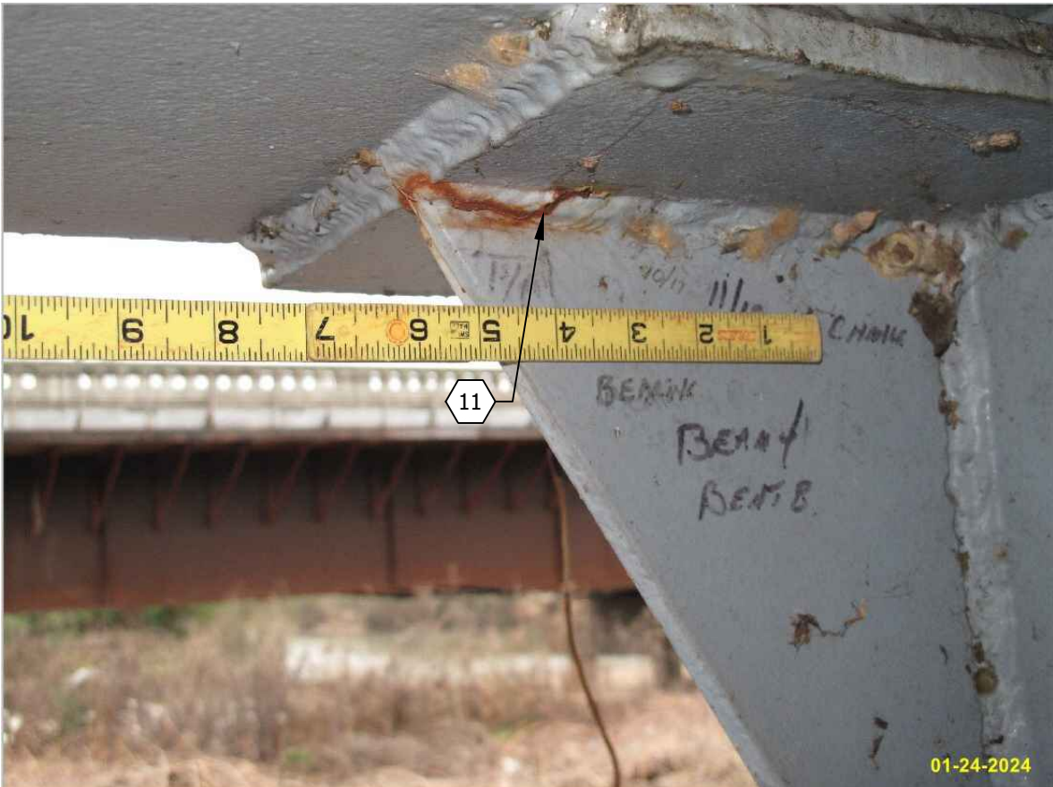
TYPICAL CRACKING OF BEARING RISER FOR GIRDERS, WEST SIDE OF GIRDER 5-4 AT BENT 5 SHOWN
