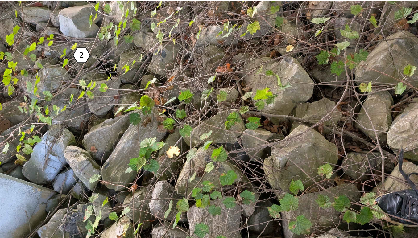
TYPICAL VEGETATION GROWTH ON RIPRAP BENEATH BRIDGE
