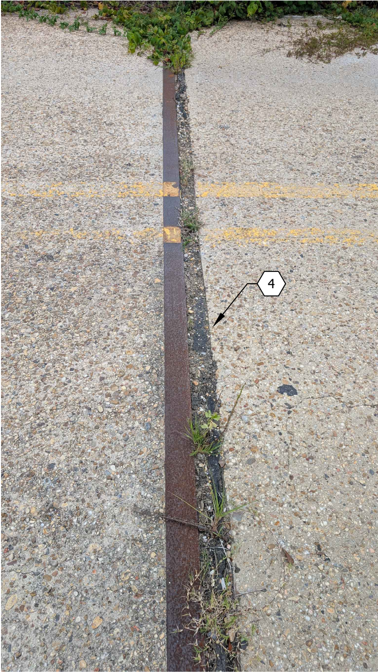
JOINT SEAL FAILURE AT METAL JOINT
