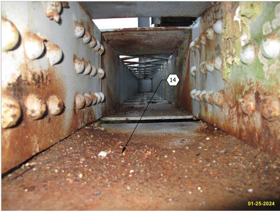
TYPICAL DEBRIS ACCUMULATION ON BOTTOM FLANGES OF LOWER CHORD
