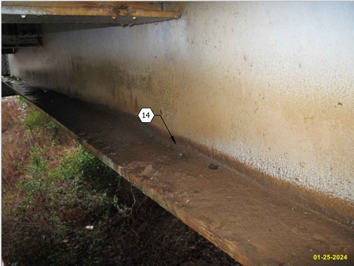
TYPICAL DEBRIS ACCUMULATION ON BOTTOM FLANGES OF FLOOR BEAM, WEST FACE OF FLOOR BEAM 1 IN SPAN 5 SHOWN
