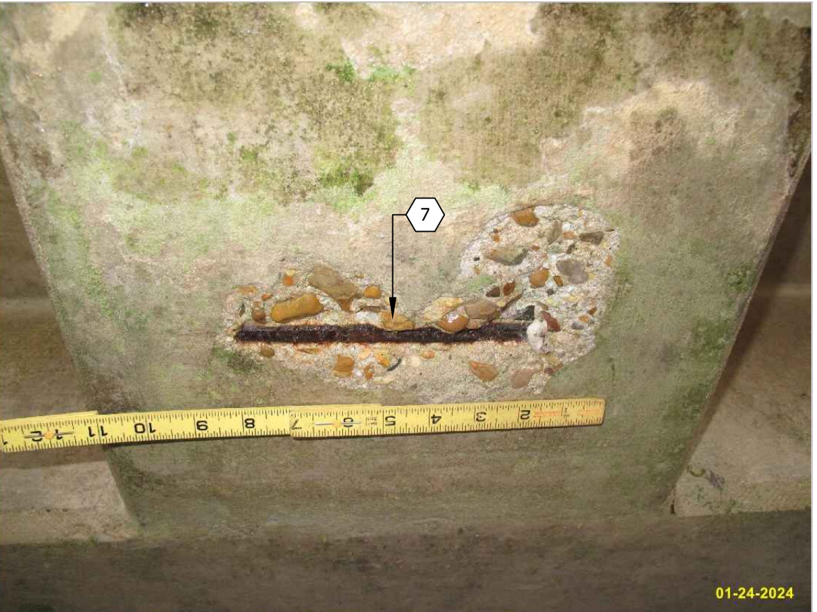
SPALLING WITH EXPOSED REBAR WITH SECTION LOSS IN BOTTOM OF CORBEL, 3RD CORBEL FOR SPAN 12 ON WEST SIDE SHOWN
