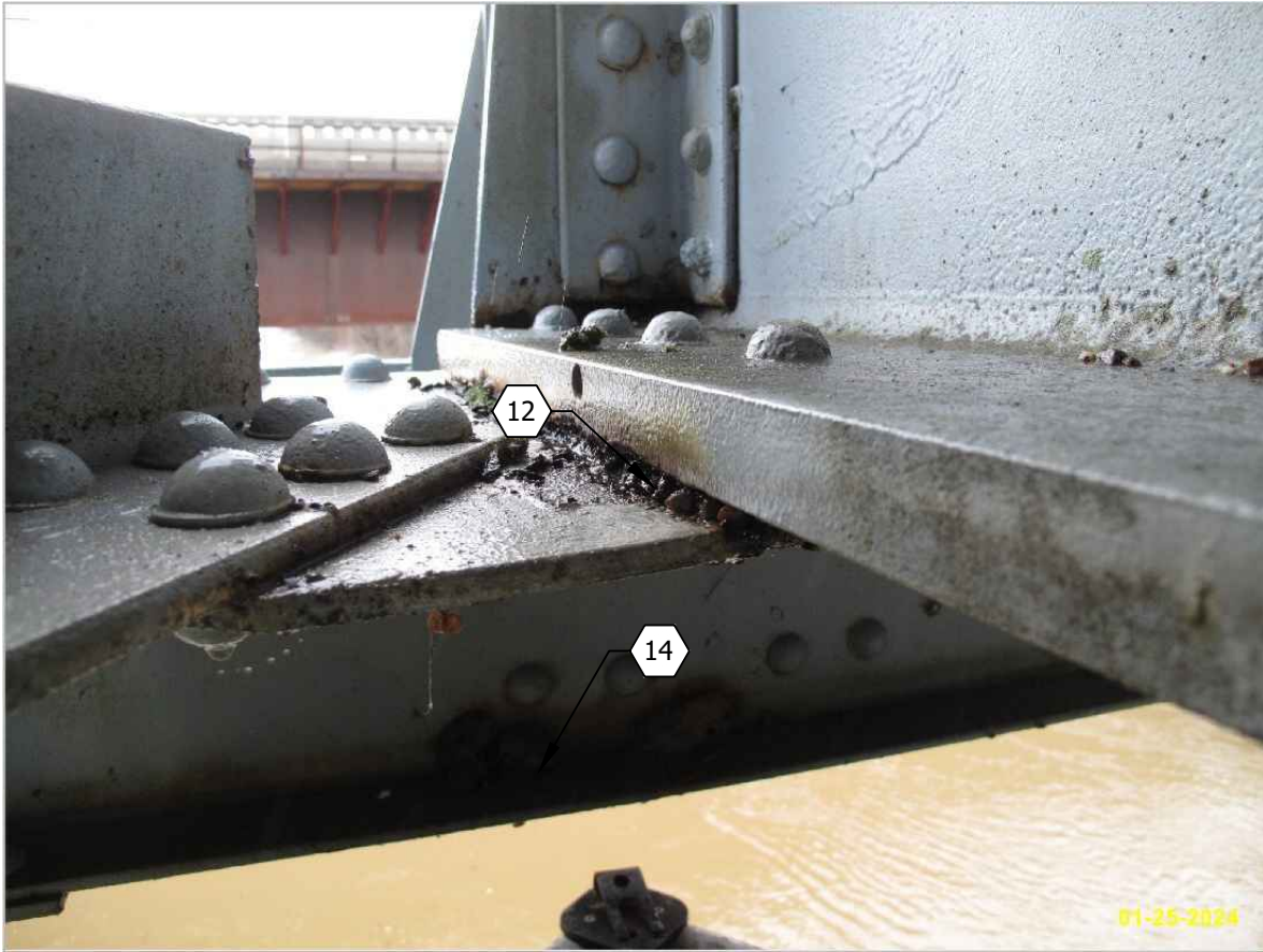
PACK RUST WITH CORROSION AND SECTION LOSS ON LOWER GUSSET PLATE FOR FLOOR BEAM 5 AND LATERAL BRACING BETWEEN FLOOR BEAMS 5 AND 6 AT EAST SIDE OF TRUSS
