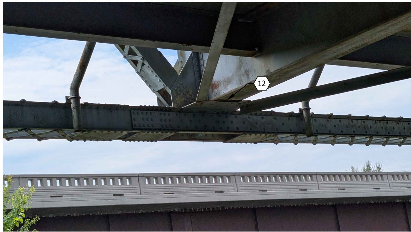
DETERIORATION OF ENCASEMENT IN BENT 5
