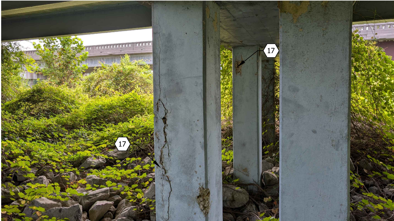
DETERIORATION OF ENCASEMENT IN BENT 5
