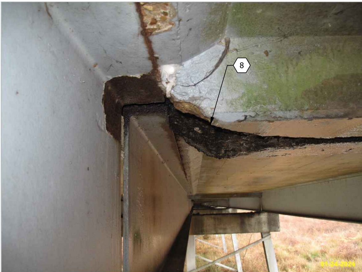
TYPICAL SPALLING OF DROP SLABS AT DECK JOINTS, JOINT AT BENT 18 SHOWN
