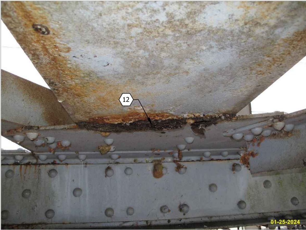
TYPICAL PAINT FAILURE, CORROSION, AND PACK RUST BETWEEN LOWER HORIZONTAL GUSSET PLATE CONNECTIONS TO FLOOR BEAMS, JOINT L13 ON EAST SIDE OF TRUSS IN SPAN 6 SHOWN
