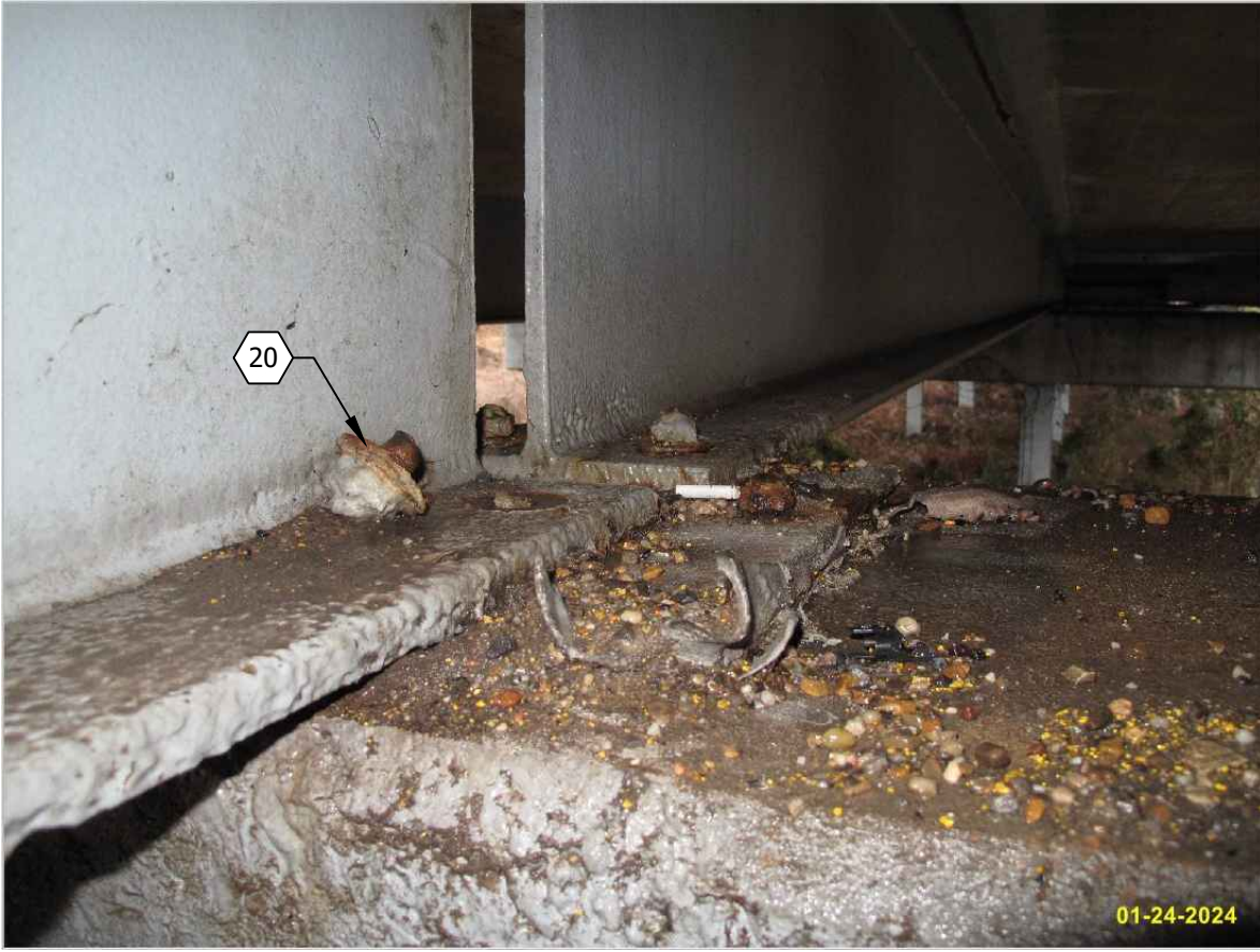
BROKEN ANCHOR BOLT FOR WEST FACE OF GIRDER 9-2 AT BENT 9
