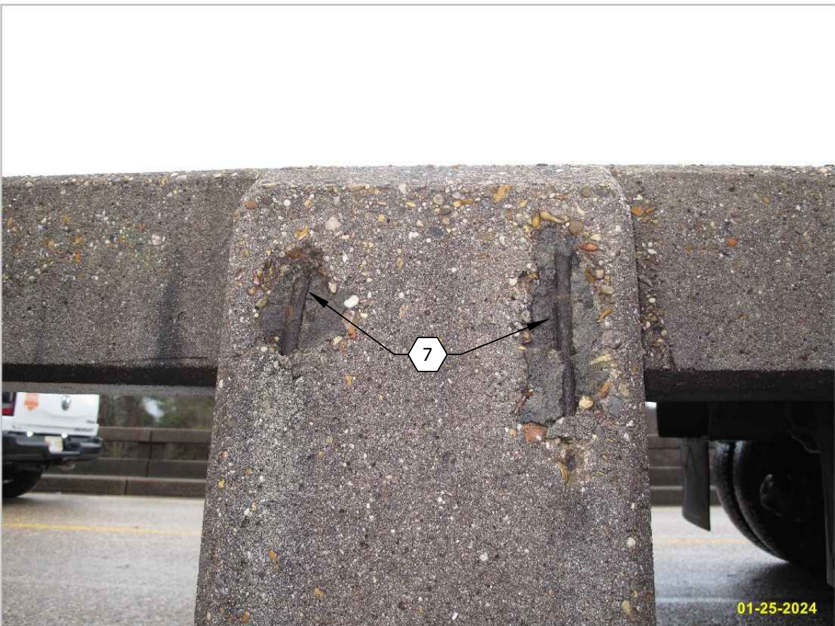
SPALLING WITH EXPOSED REBAR DUE TO INSUFFICIENT COVER ON 3RD AND 4TH BRIDGE RAIL POSTS FOR EAST BRIDGE RAIL IN SPAN 12, 3RD POST SHOWN
