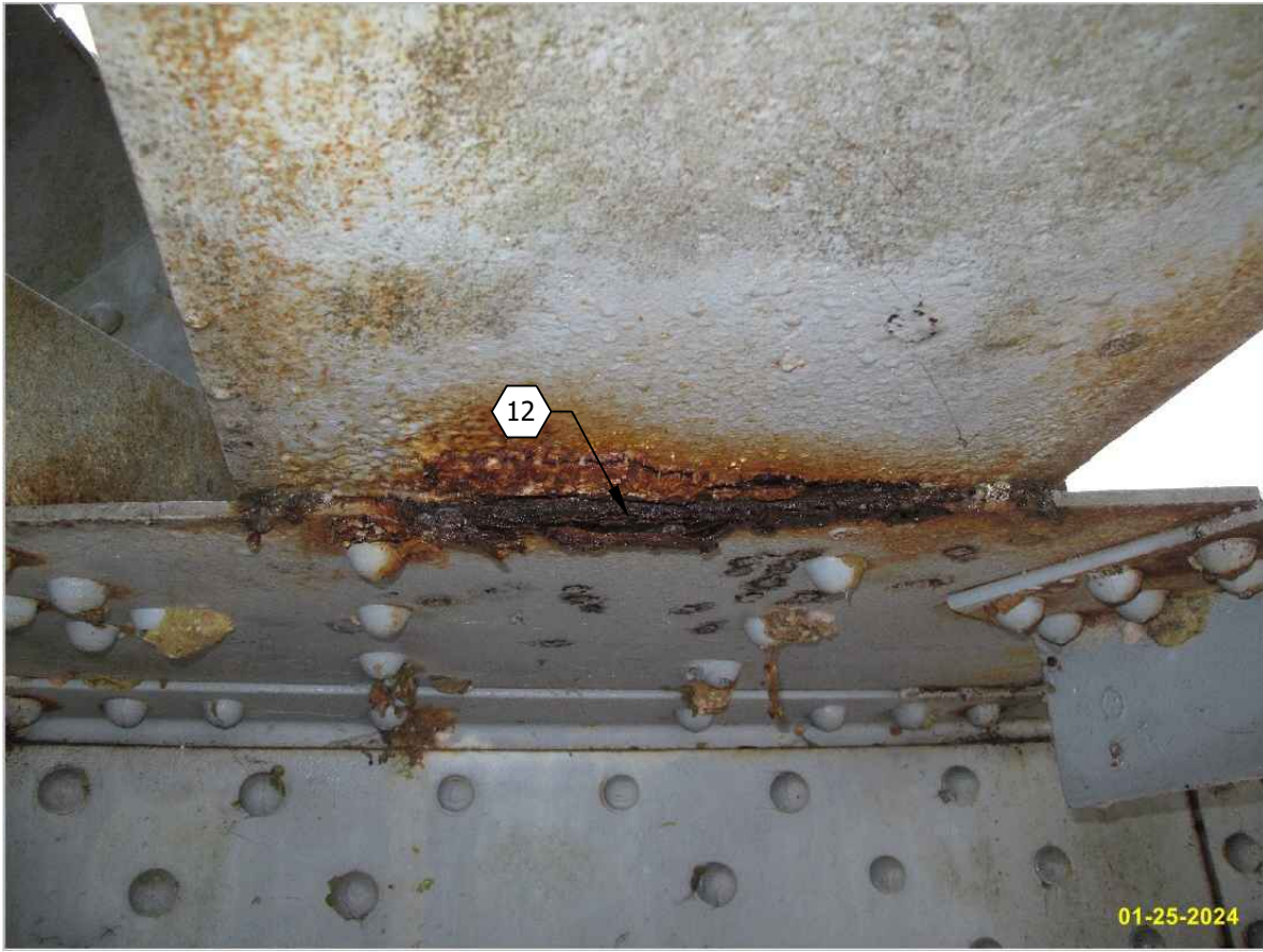
TYPICAL PAINT FAILURE, CORROSION, AND PACK RUST BETWEEN LOWER HORIZONTAL GUSSET PLATE CONNECTIONS TO FLOOR BEAMS, JOINT L12 ON EAST SIDE OF TRUSS IN SPAN 6 SHOWN
