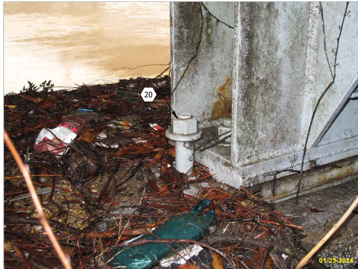
LOOSE ANCHOR CONNECTION HARDWARE ON BEARING FOR GIRDER 4-1 AT PIER I
