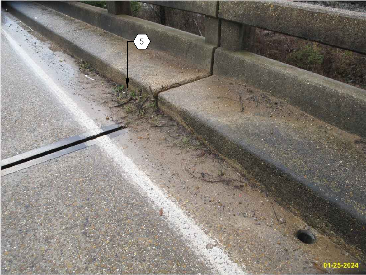
TYPICAL JOINT SEAL FAILURE, BENT 6 JOINT SHOWN
