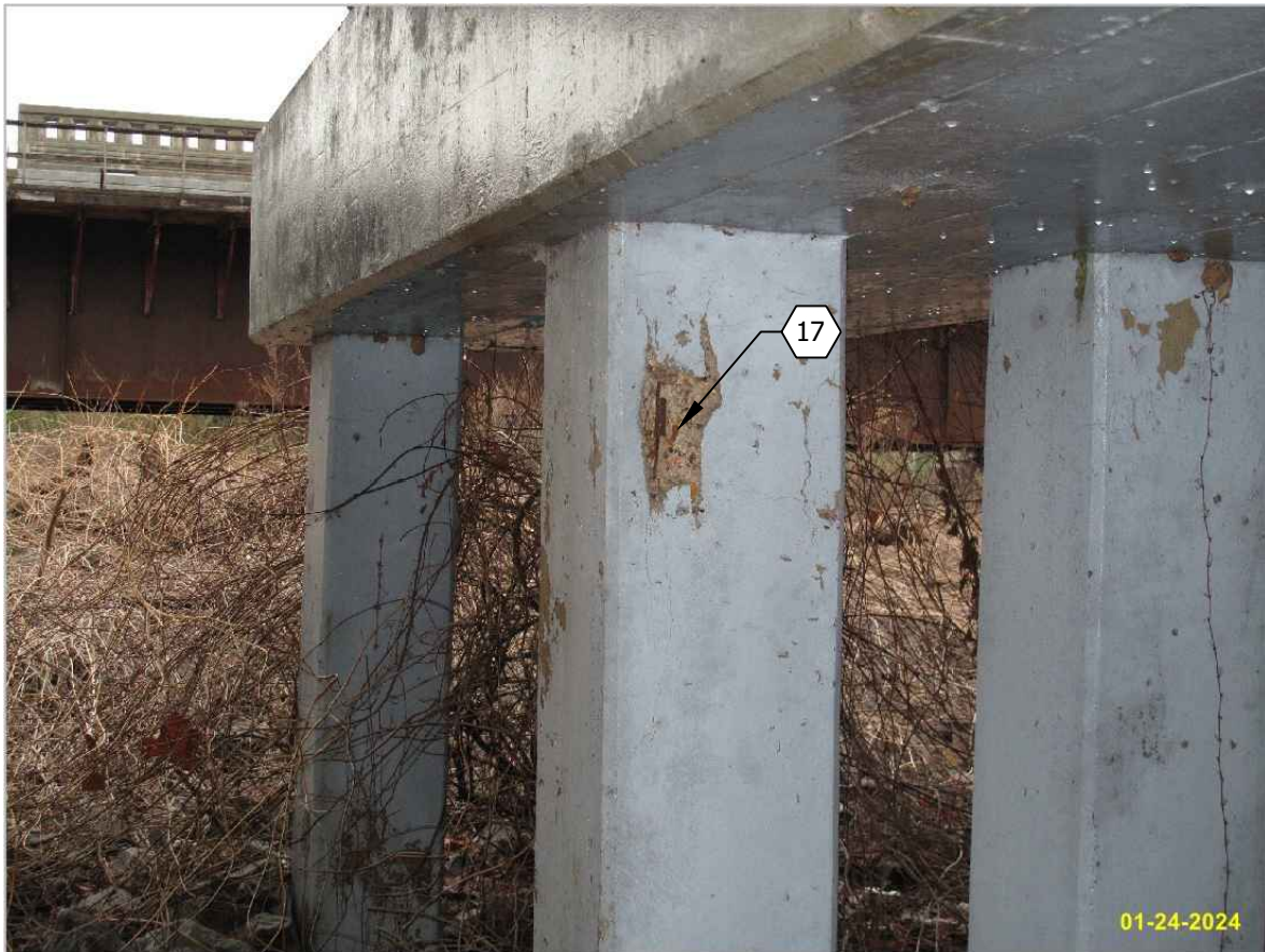
TYPICAL CRACKING, DELAMINATION, AND SPALLING OF CONCRETE PILES, PILE 5-38 SHOWN
