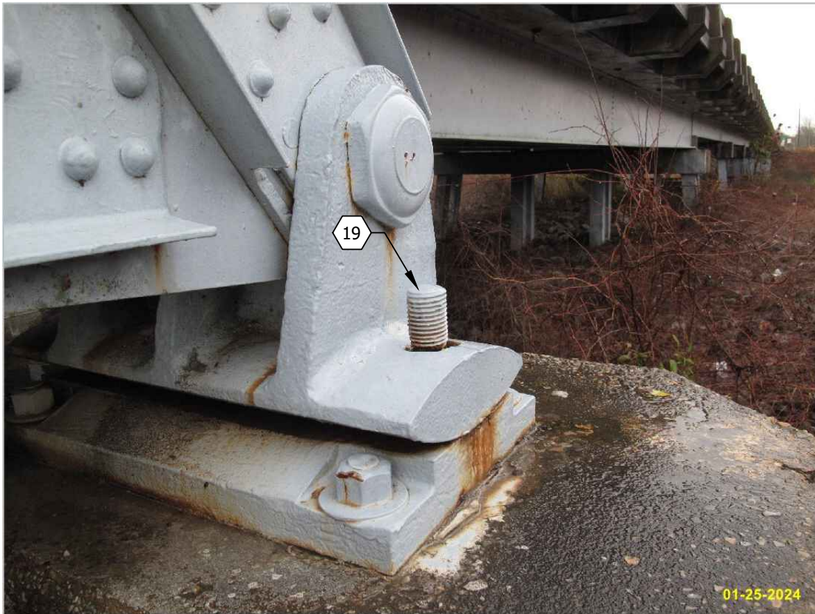
MISSING EXTERIOR CONNECTION HARDWARE FROM EAST ROCKER BEARING AT PIER III
