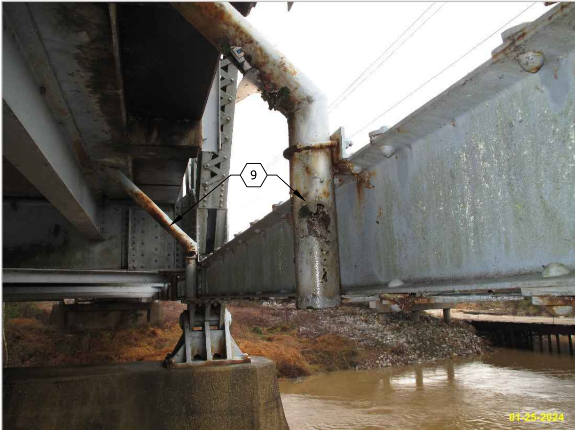
TYPICAL SPALLING ON DECK OVERHANG, STRINGER 6 FOR SPAN 6 BETWEEN L1' AND L2' SHOWN
