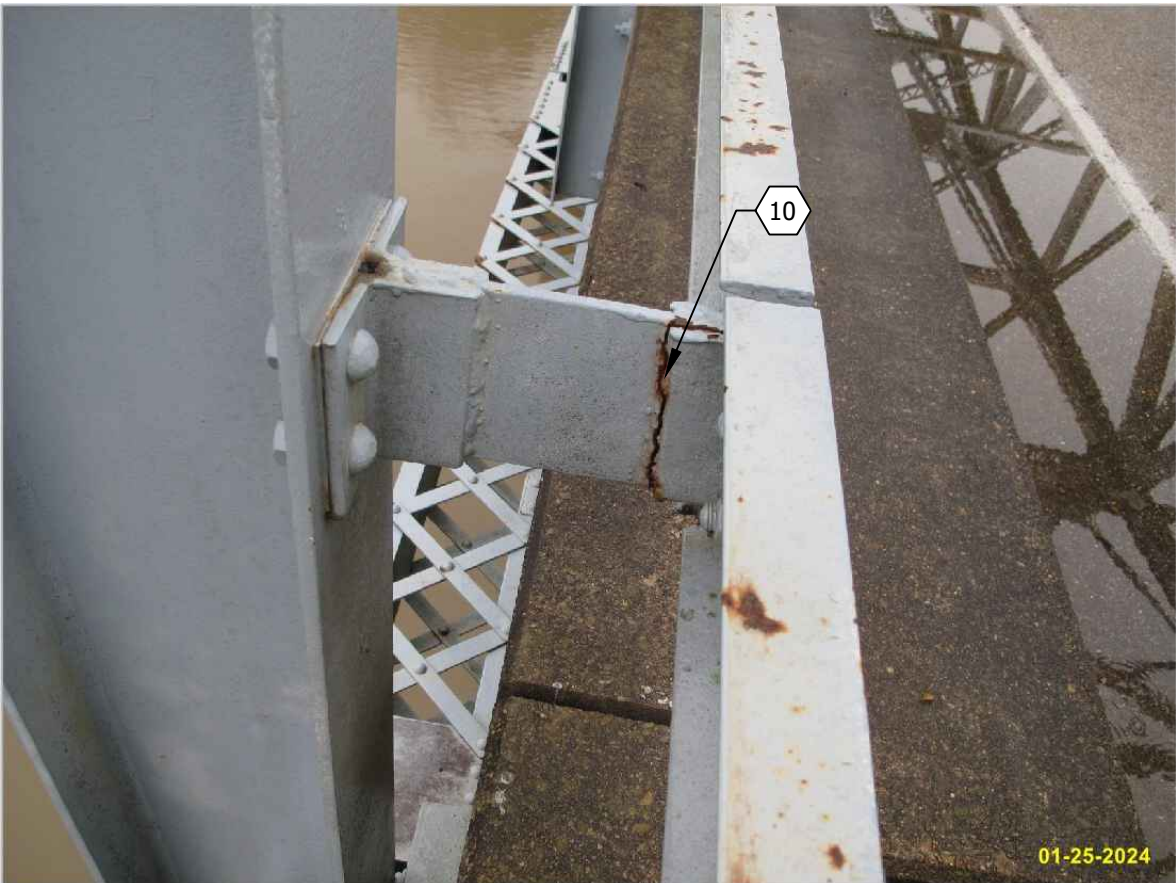
BROKEN WELD CONNECTION FOR WEST BRIDGE RAIL AT U5-L5
