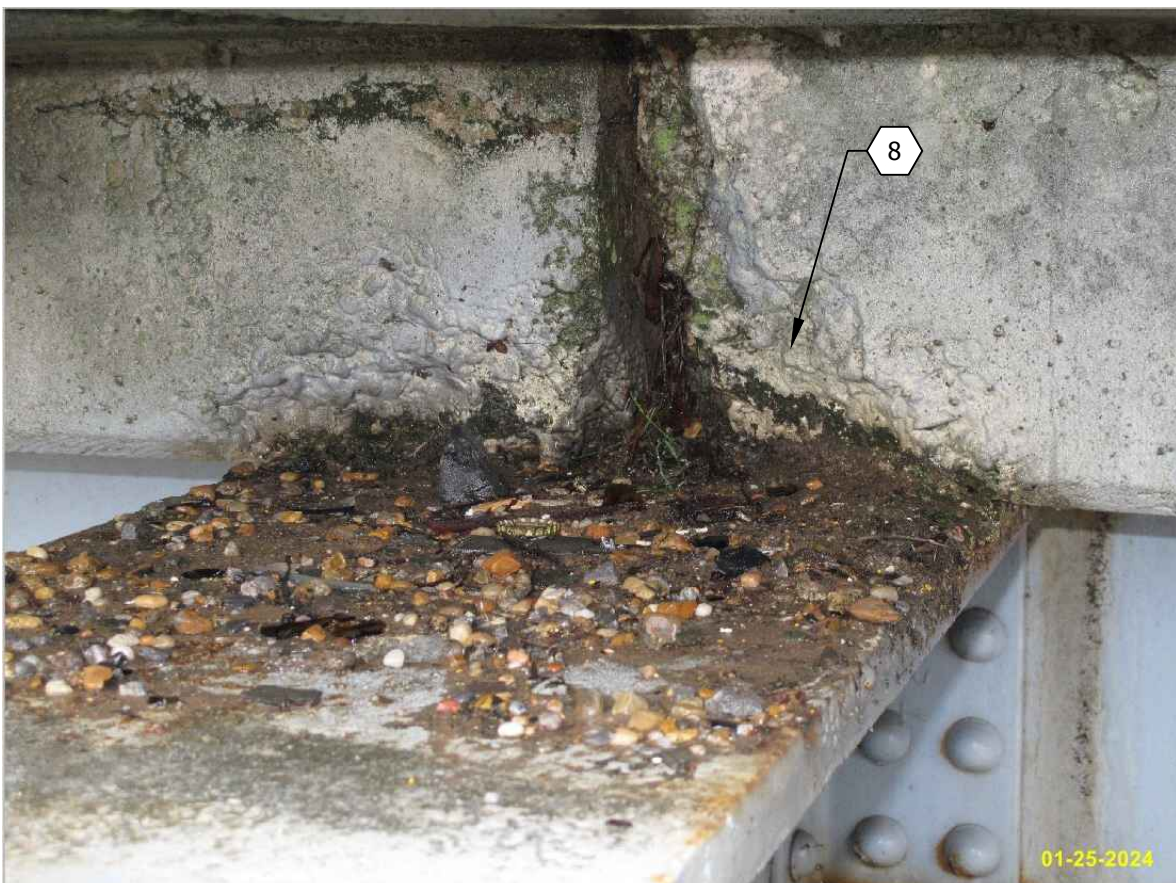
TYPICAL SPALLING OF DROP SLABS AT DECK JOINTS, JOINT AT L6 FOR SPAN 5 SHOWN
