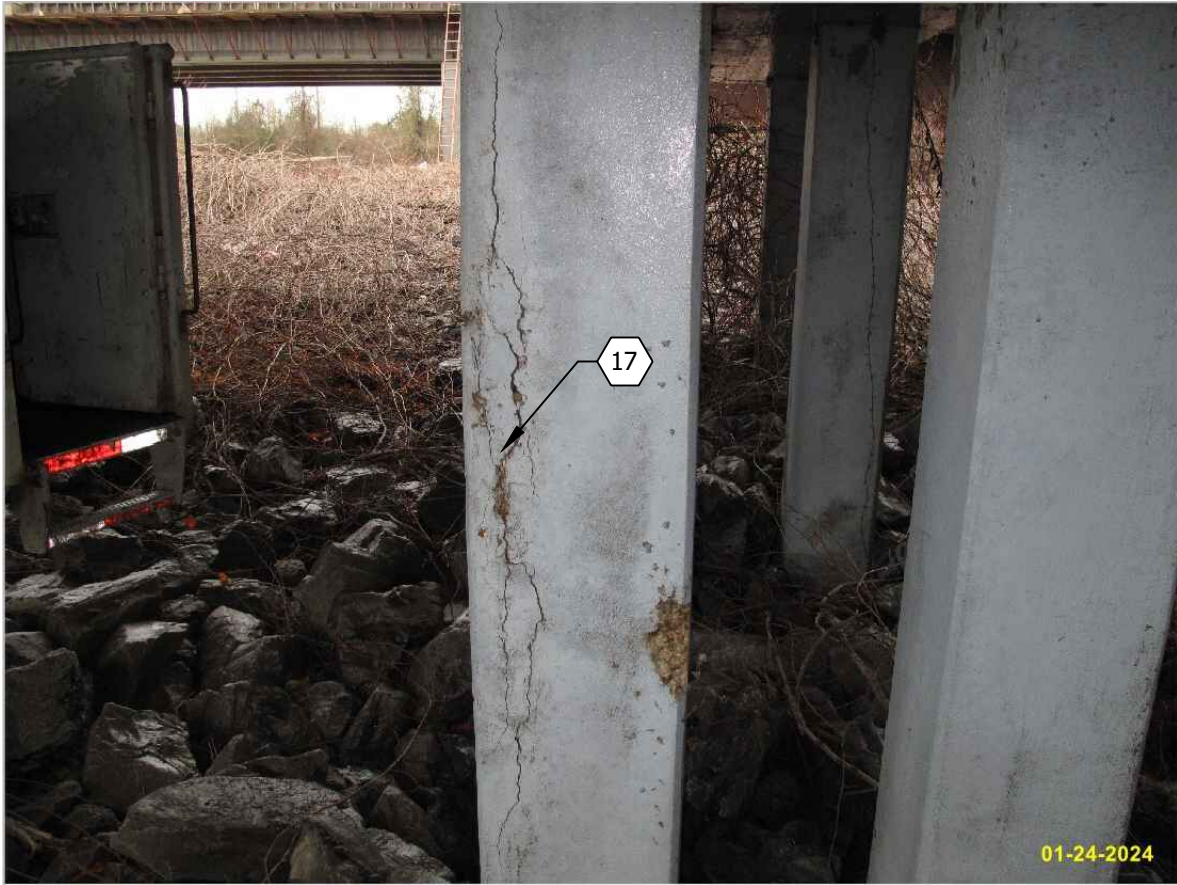
TYPICAL CRACKING, DELAMINATION, AND SPALLING OF CONCRETE PILE ENCASEMENT, PILE 5-28 SHOWN
