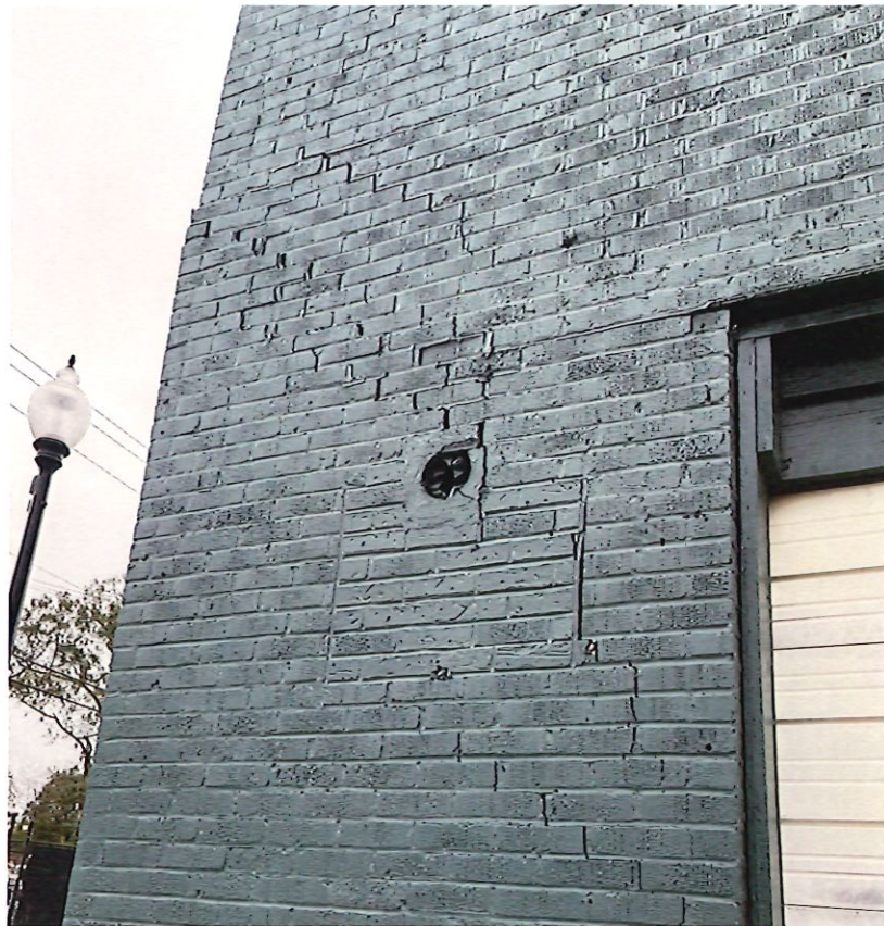
SW Corner (top) and east wall (below)—step cracking in masonry
