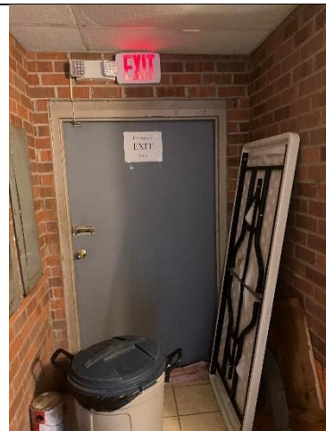
Rear Exit Door
