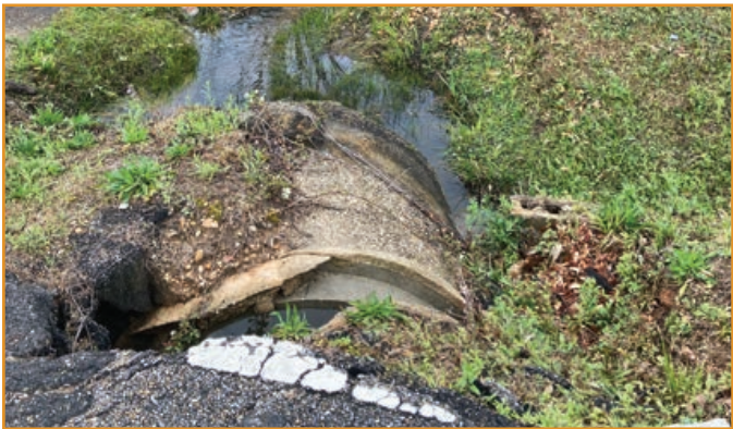
F Erosion at culvert crossings
