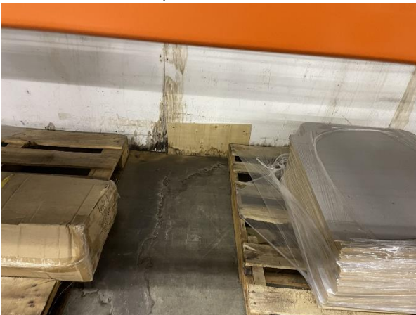
View of water damage in warehouse Picture taken on October 5, 2022
