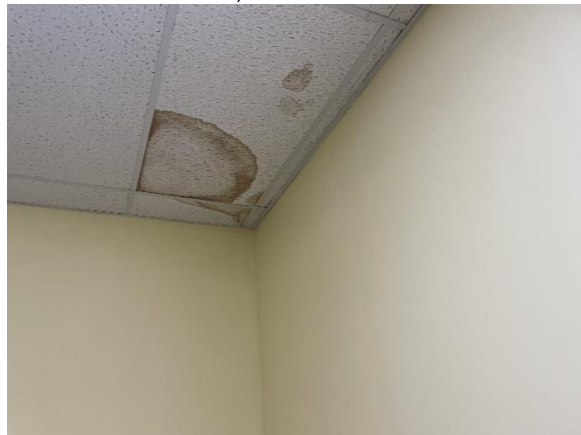
View of water damage on ceiling Picture taken on October 5, 2022
