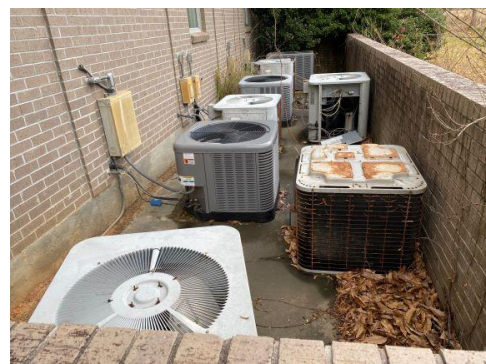
HVAC units in front of building
