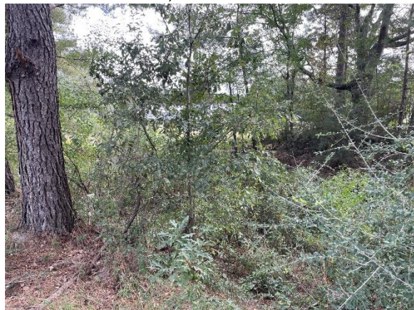
View of overgrown drainage ditch Picture taken on October 5, 2022
