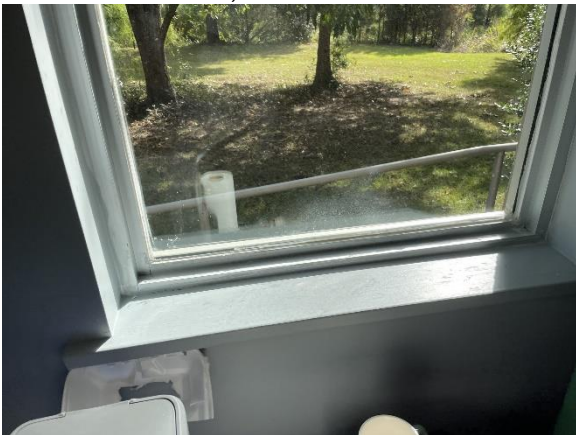
View of repaired window with leaks Picture taken on October 5, 2022
