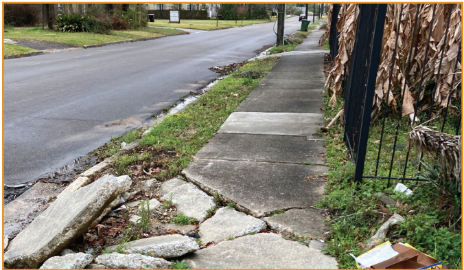
K Broken and discontinuous sidewalks along south end of N 25th Ave
