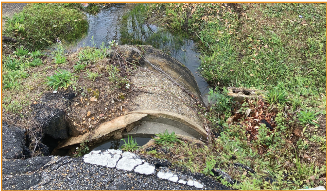
F Erosion at culvert crossings
