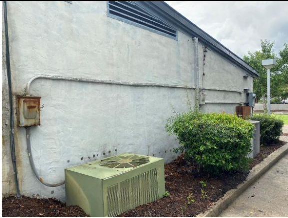
HVAC units located on the north side of the building
