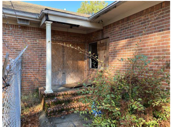
Deferred maintenance at the rear of the building
