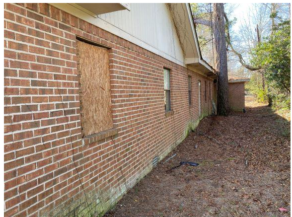
Deferred maintenance on the west side of the building.
