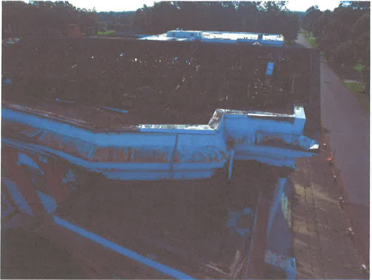
Figure 2 Roof Condition Southwest Corner Facing Main Street
