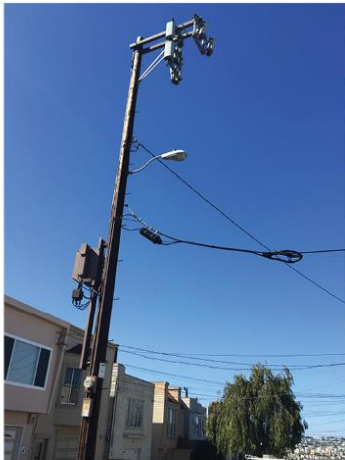
Poor installation plan with antenna and equipment protruding from pole and wiring visible at accessory equipment.
