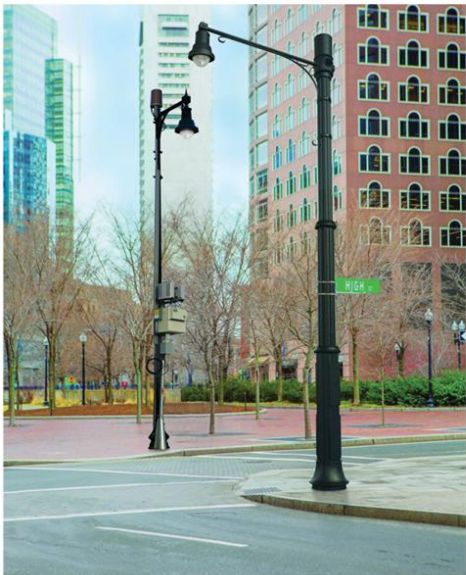
Foreground shows a decorative pole with all equipment fully concealed within the base of a pole. Background shows a similar decorative pole but with equipment installed in a prohibited manner. Equipment should be concealed within the pole or installed at ground level in an appropriate location or underground, and wiring should be completely concealed.
