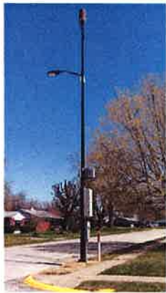
Effective small cell, light pole combination except that equipment may need to be elevated and wiring concealed.
