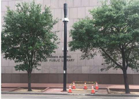
Effective monopole sample with the exception of wiring being visible at equipment connections and that all equipment meet the color requirement.
