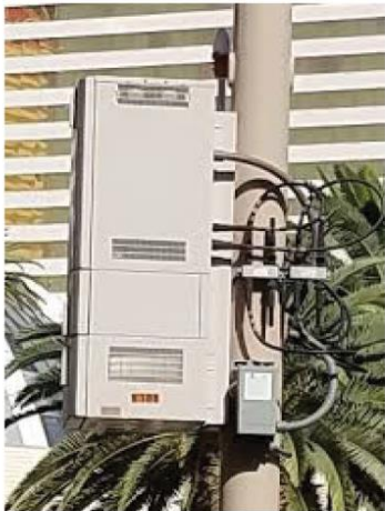
Poor installation with wiring visible.
