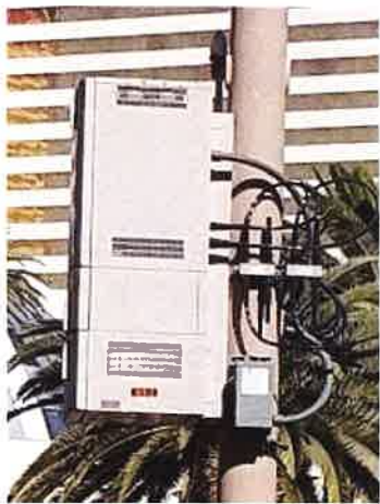
Poor installation with wiring visible.
