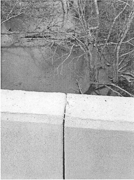
Figure 3: Spall on railing
