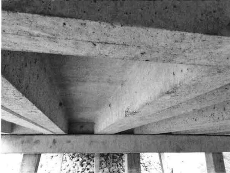
Figure 1: Spalls on underside of span units
