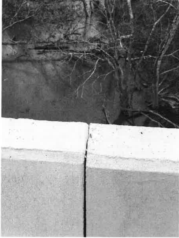
Figure 3: Spall on railing
