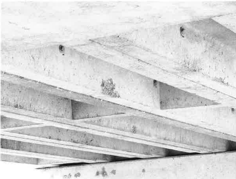
Figure 2: Spalls on underside of span unit
